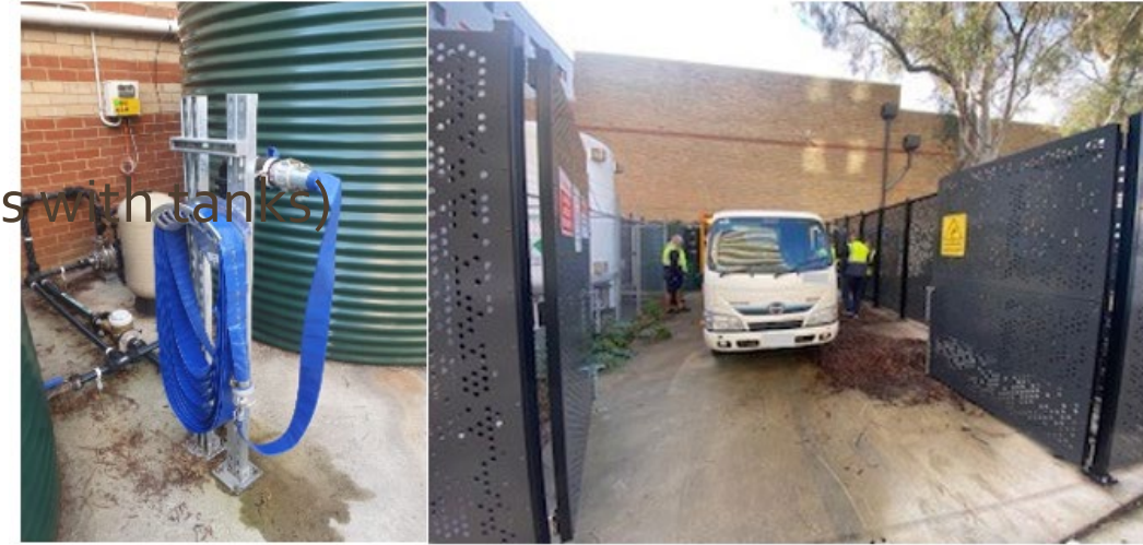
Figure 6(a)(b) - Original hose setup and water collecting spot in July 2023
