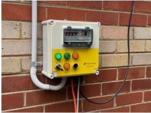
(c) – Pump controller
